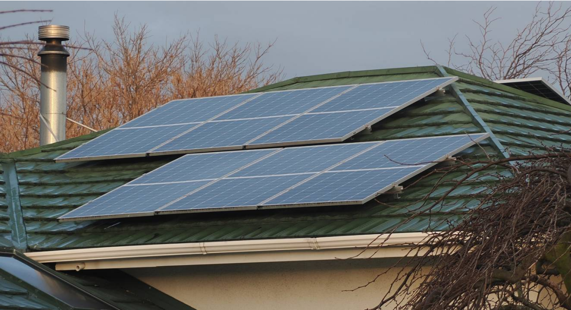
Solar electricity (solar panels, photo-voltaics, PV)
